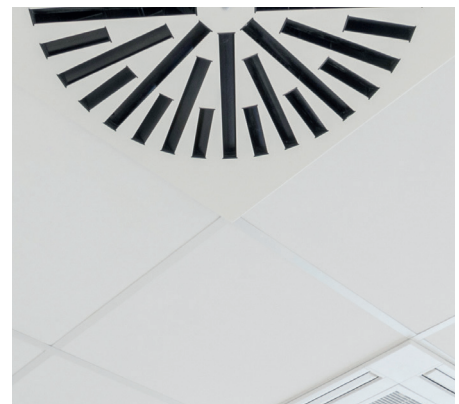
Air conditioning built into the suspended ceiling grid
