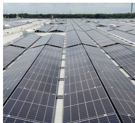
Large-scale PV system for electricity generation
